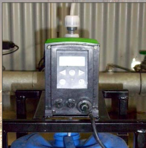
Water treatment unit
